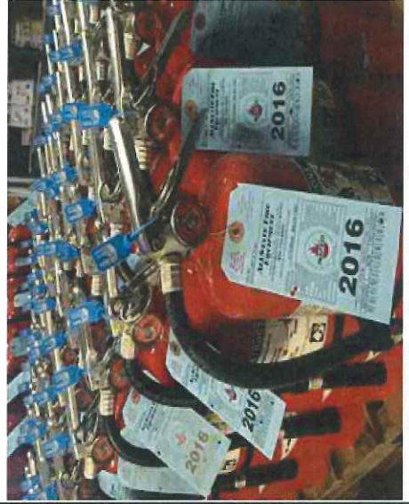
Tagged and inspected fire extinguishers done annually.
