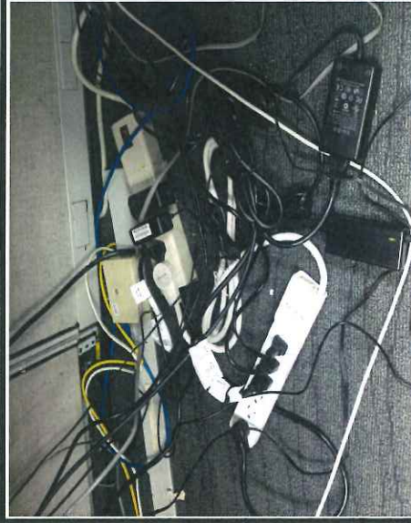
Daisy chained surge strips.
